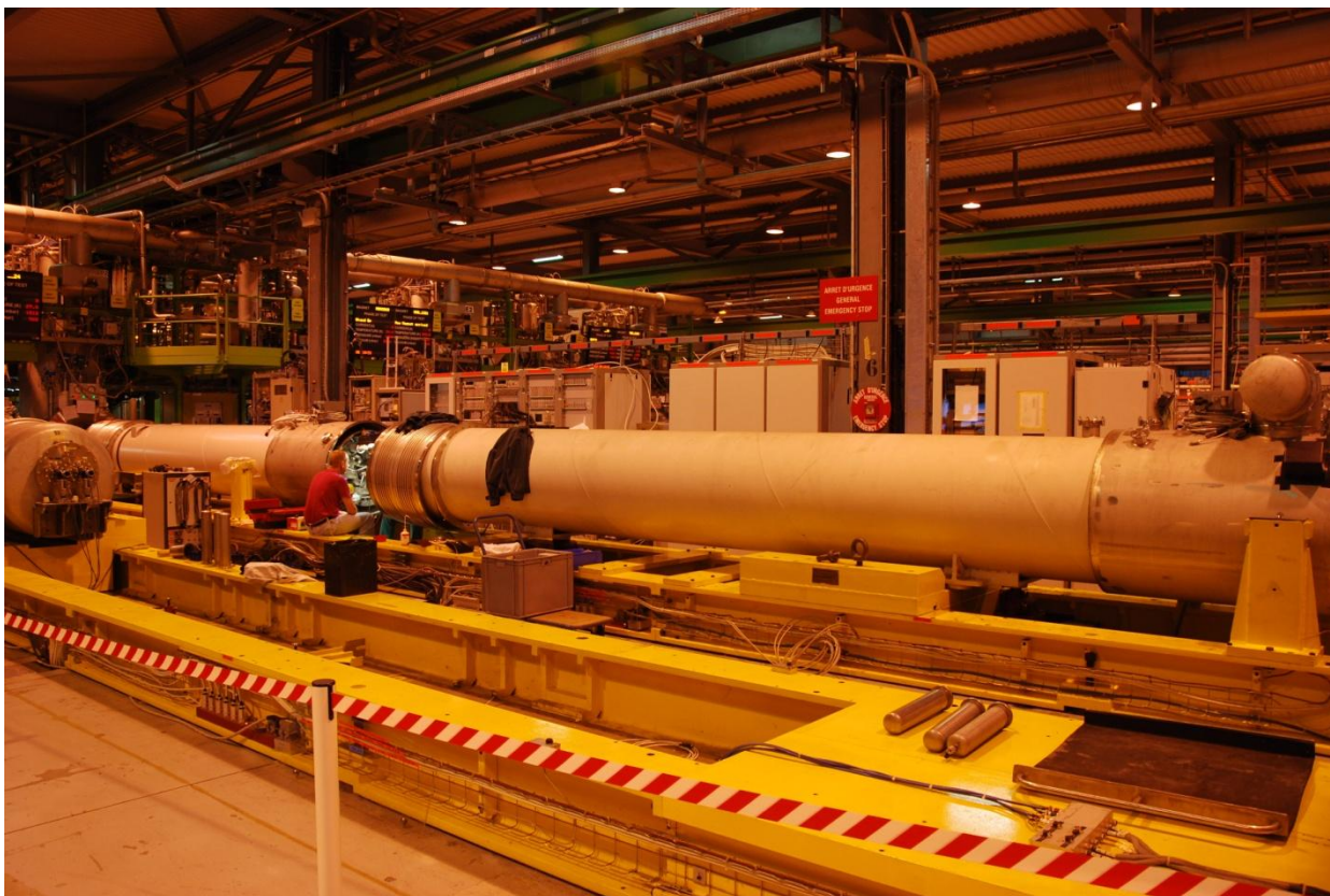
Figure 48. Overview of the Q8 and Q9 positioned on the test bench
