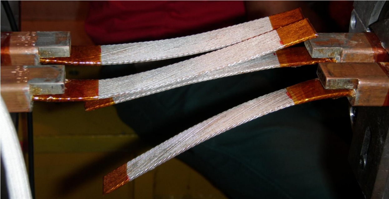
Figure 32. M3 interconnection region with the cables from the Q8 and Q9 cold mass still disconnected. The Polyimide tape is wound around the cable to create the non-stabilized cable length, or defect length.
