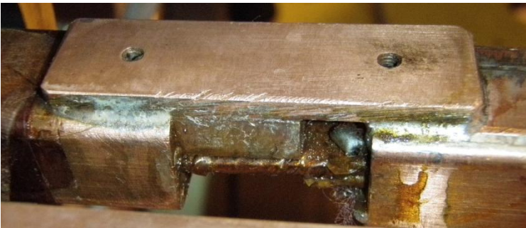
Figure 38. Close up of shunt 2 in interconnection M3b
