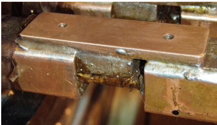
Figure 35. Close up of shunt 1 in interconnection M3a
